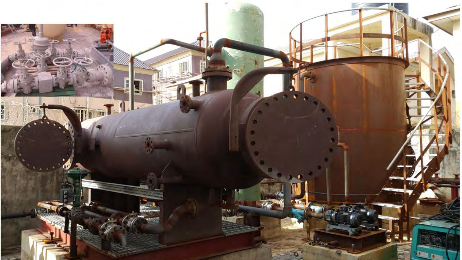
FEDP Pilot Oil and Gas Surface Production Facility having Wellhead, Flowline, Inlet Manifold, 3-Phase Separator, Surge Vessel, Piping, Tank, Transfer and Export Pumps, Pipeline, Pig Launcher/Receiver and Produced Water Treatment
